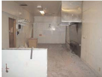
Kitchen has plumbing, venting & electric in place for a commercial kitchen. Also has an ansef fire suppression system.
